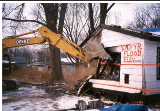
This home in Lake County was not worth relocating, so it was acquired and demolished by the County. The site is now open space.
