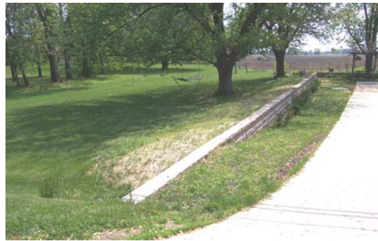
This barrier in Otto Township protects the home from flooding from the stream to the left.
